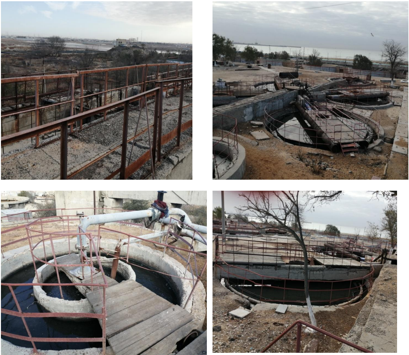
Figure 1. – Condition of the wastewater treatment facilities in Aktau
